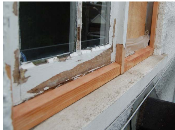
Garden Village windows under repair in 2015 Picture courtesy of Lazron Matia Preservation Joinery (02921 328090 07843257616 laz.matia@gmail.com)
