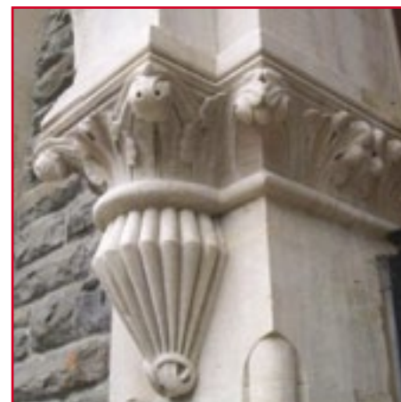
Bath stone pilaster topped by an ornately carved capital and corbel - doorway at 3 Park Place.
