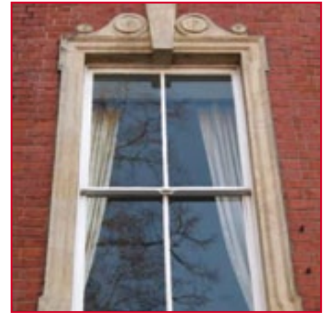
Windsor Place – first floor sash window with classical detailing in Bath stone
