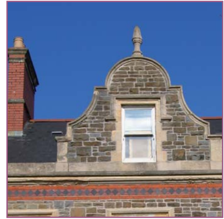
Dutch styled gable with a timber framed sash window and sandstone walling, Windsor Esplanade
