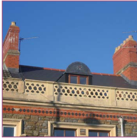
Round headed attic dormer, red brick chimneys and bathstone detailing, Windsor Esplanade
