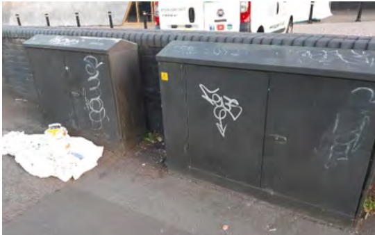
Utility Boxes with Graffiti
