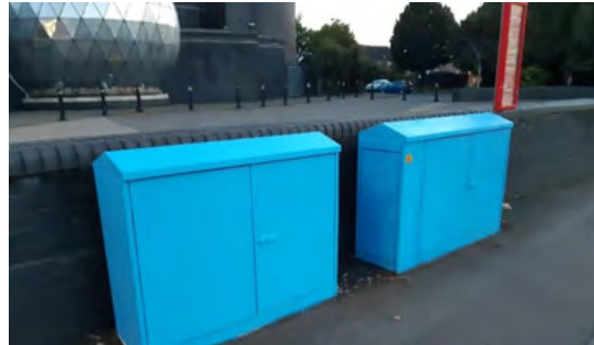
Utility Boxes after Graffiti Removal Team
